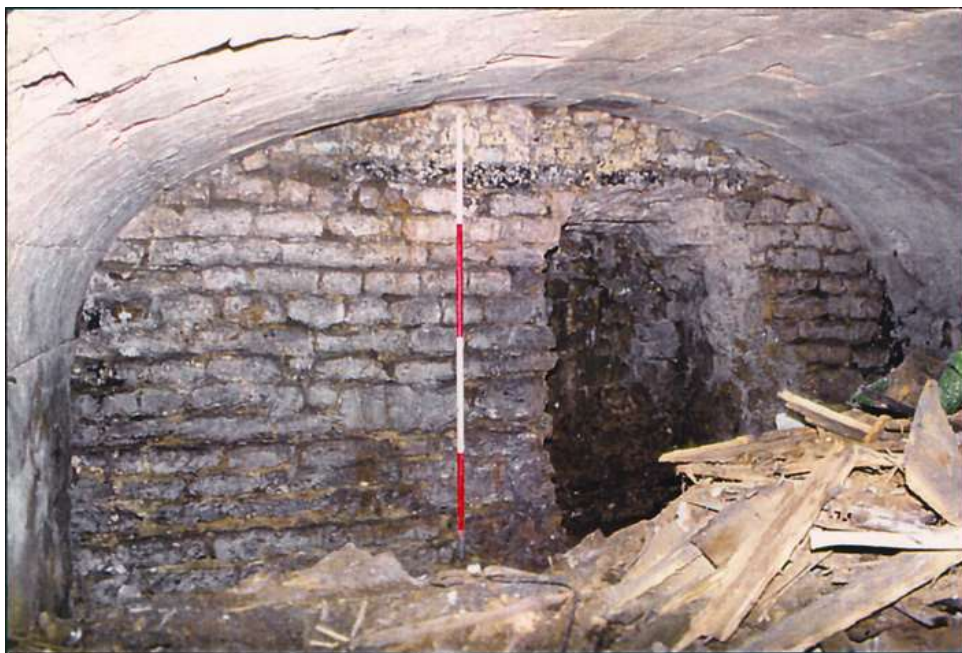
The city wall in a cellar beneath Terrace Walk. The opening on the right appears to be the result of an unsuccessful attempt to break through the wall.
